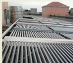
Solar Energy System
