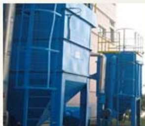
Empties Treatment System
